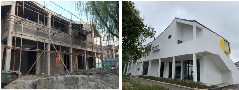
Figure 1. Image of the investigated building during construction (left); Figure 2. Image of the investigated building after construction (right)
