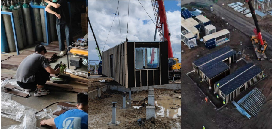
Figure 5. From left to right: students cut bamboo panels; position a module to the foundation; and the on-site assembly of five modules
