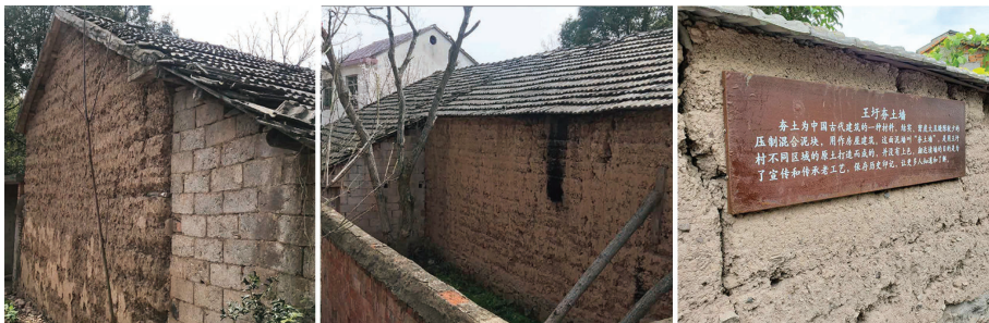
Figure 1. Status Quo of Grey Tile, Pitched Roof and Rammed Earth Wall.
